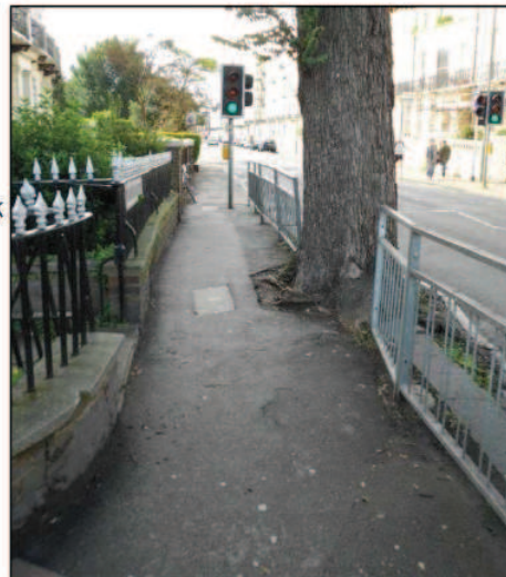
Footway width below standard 2.0m
