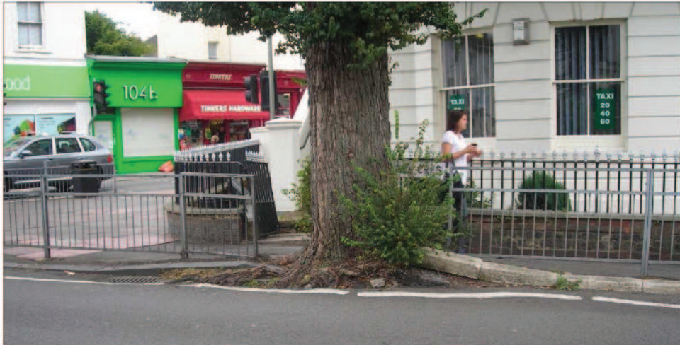
Existing carriageway and footway have been displaced / adjusted to suit the growth of the tree
